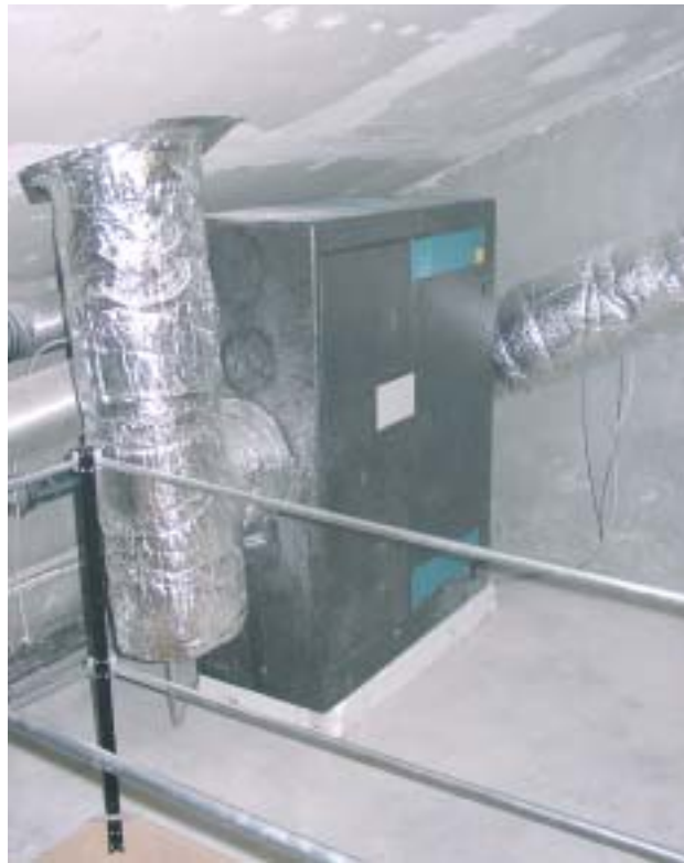
Figure 21: Ventilation unit with heat exchanger in the building services floor of a Hannover-Kronsberg Passive House. In the background is the fresh air duct with defrost heater and in the foreground is the exhaust air pipe (both insulated with mineral wool, aluminium laminated)
